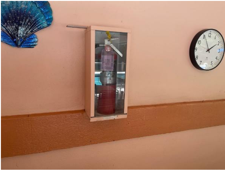
Photos / Fire Protections
